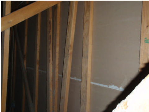
No insulation on sidewall at north side of house
