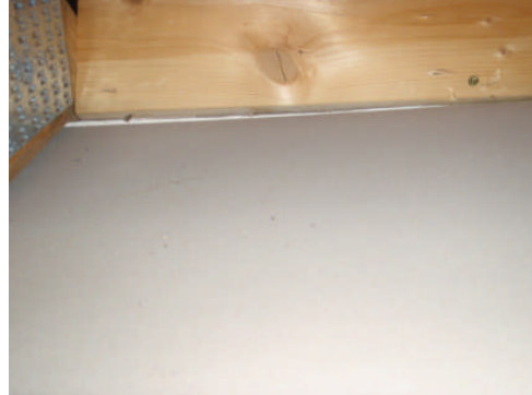
No visible insulation at peak areas
