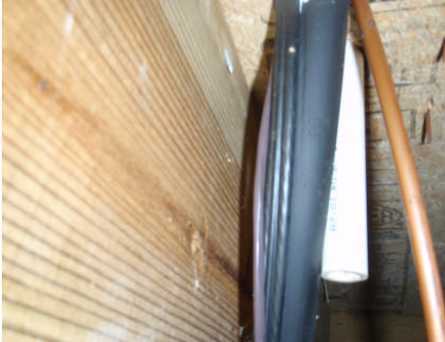
Condensation drain line (white) empties under house
