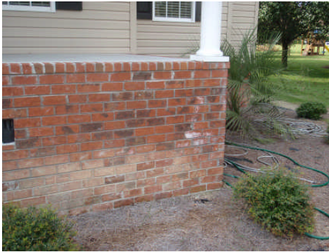
Front porch over 4' above grade
