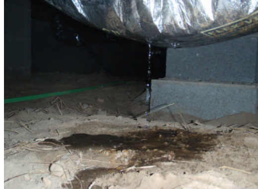
Ductwork under kitchen area full of water
